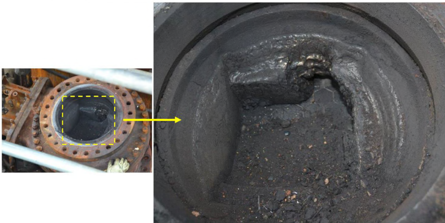
Figure 33. Spent catalyst slide valve in-situ. (Credit: Husky Superior Refinery with annotations by CSB)
