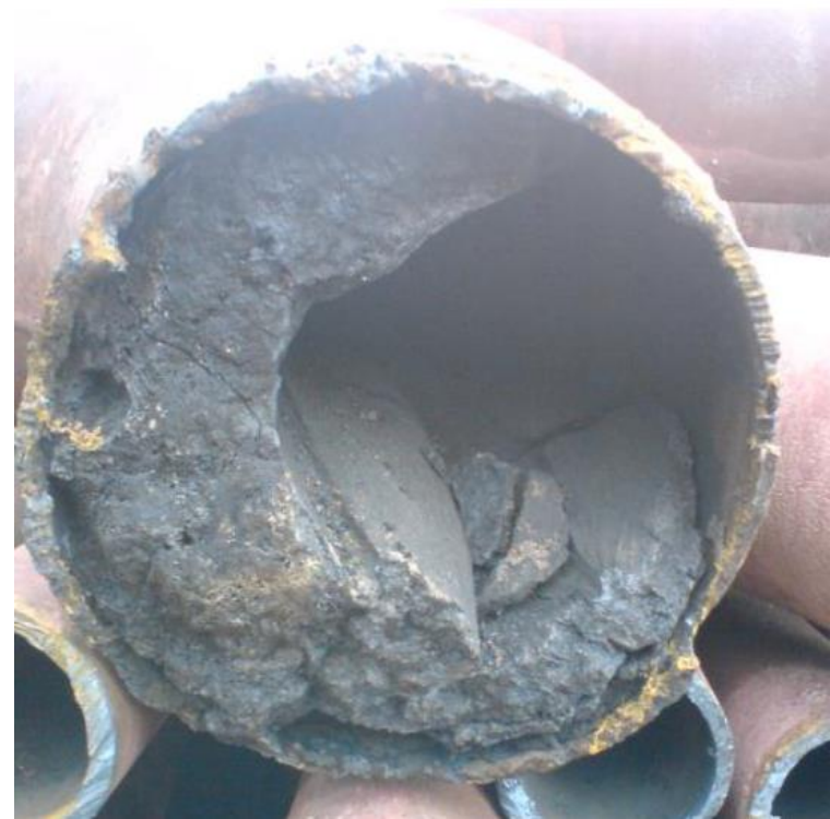
Coked Furnace Tube – U-Bend
