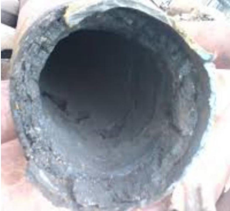
Coked Furnace Tube – Straight Run
