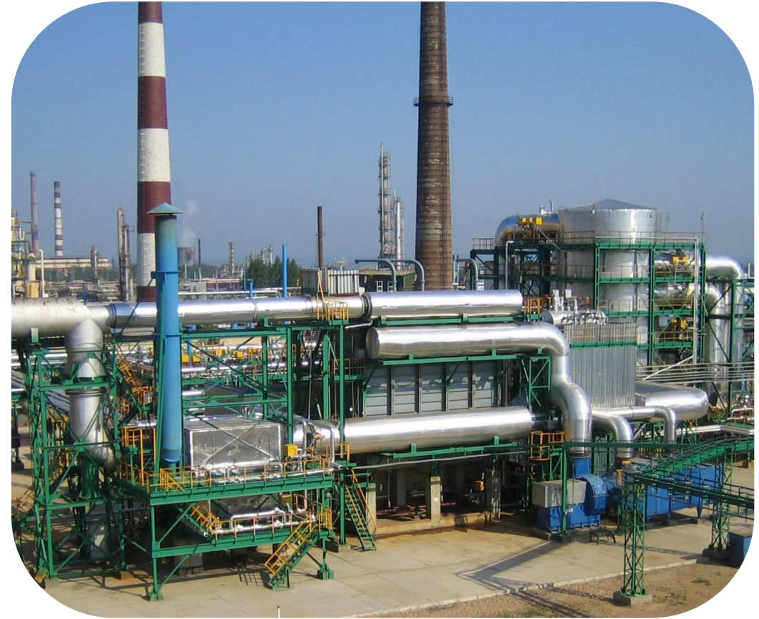
Sulfuric acid plant (WSA)
