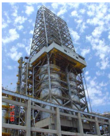
Coke Drum Switching
