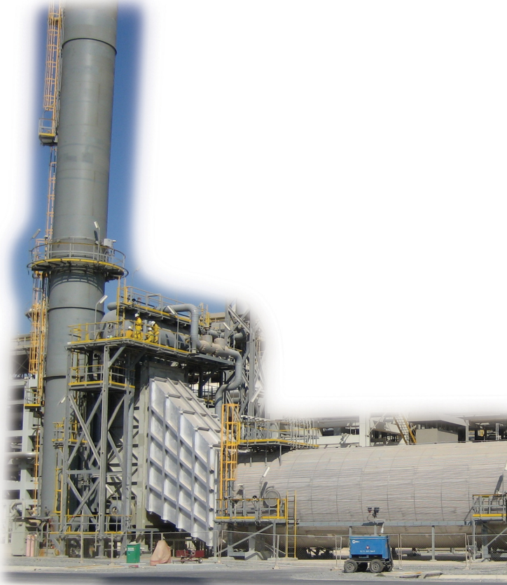
Figure 5. Tail gas incinerator with heat recovery boiler
