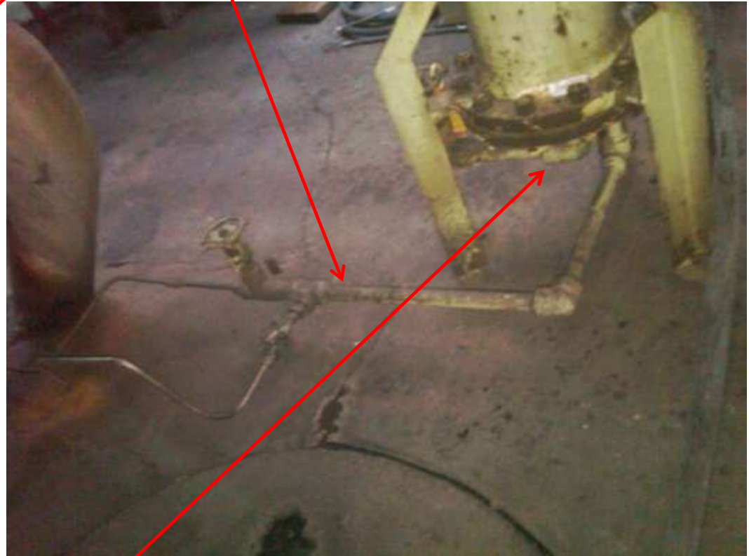
Water outlet & inlet piping from furnace
