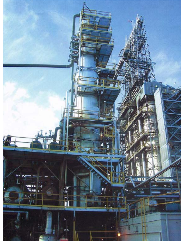
Main Fractionator Vessel
