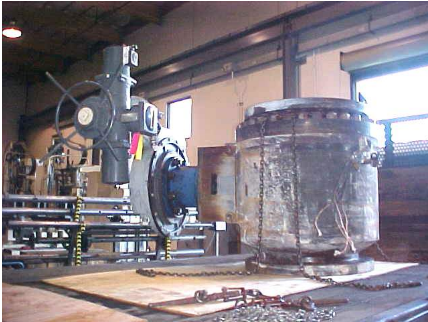
Delayed Coker Motor Operated Valves
