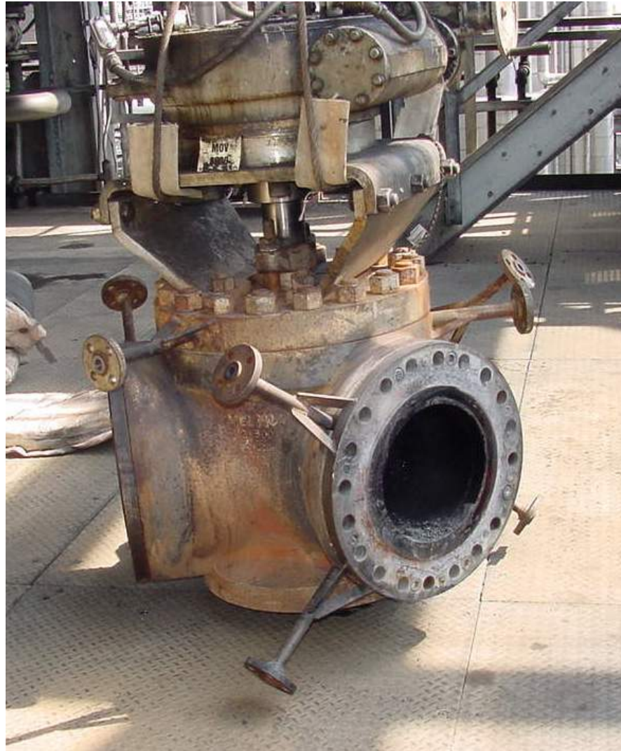
Delayed Coker Motor Operated Valves
