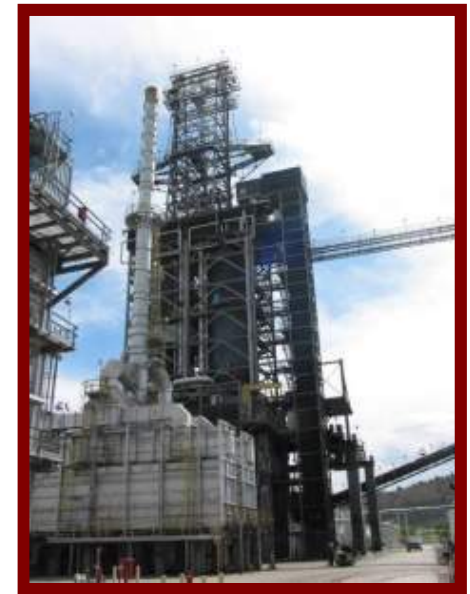
Billings Refinery Coker Courtesy of CoP
