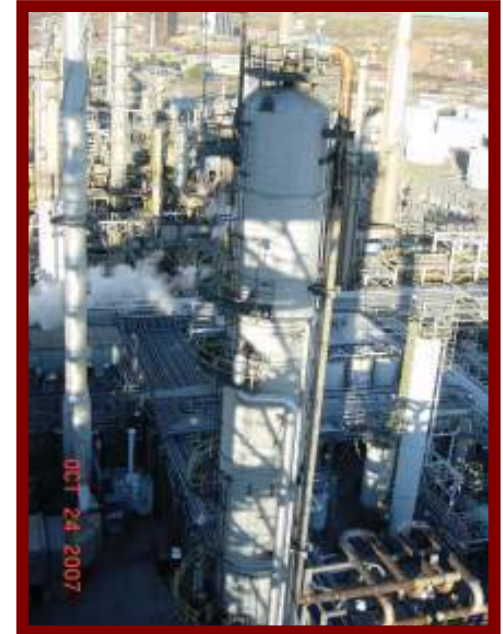
Billings Refinery Coker Courtesy of CoP
