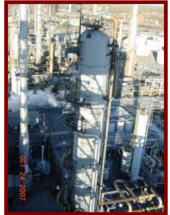
Billings Refinery Coker Courtesy of CoP
