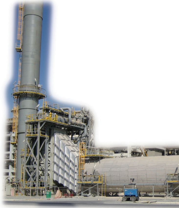
Figure 5. Tail gas incinerator with heat recovery boiler
