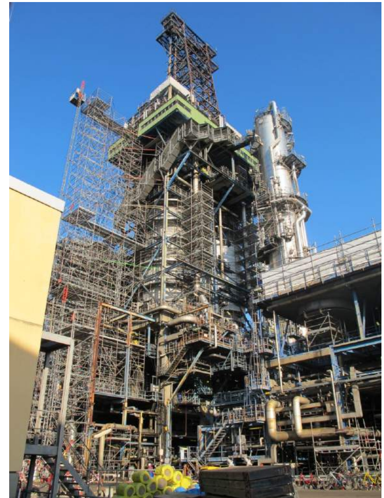
Delayed Coking Unit
