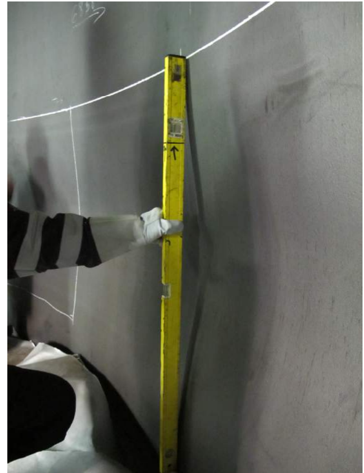
Shell Bulging Damage
