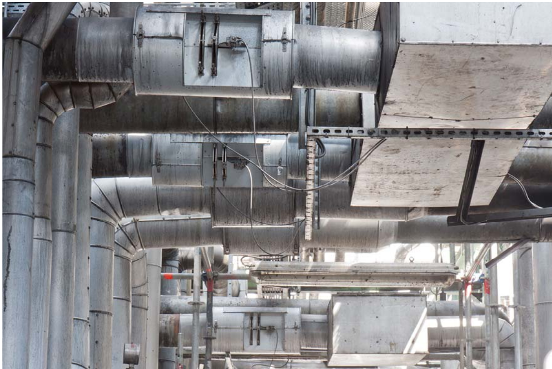
Fig. 24 : WaveInjectors® Insulated at the Feed Lines of the Coker Furnace
