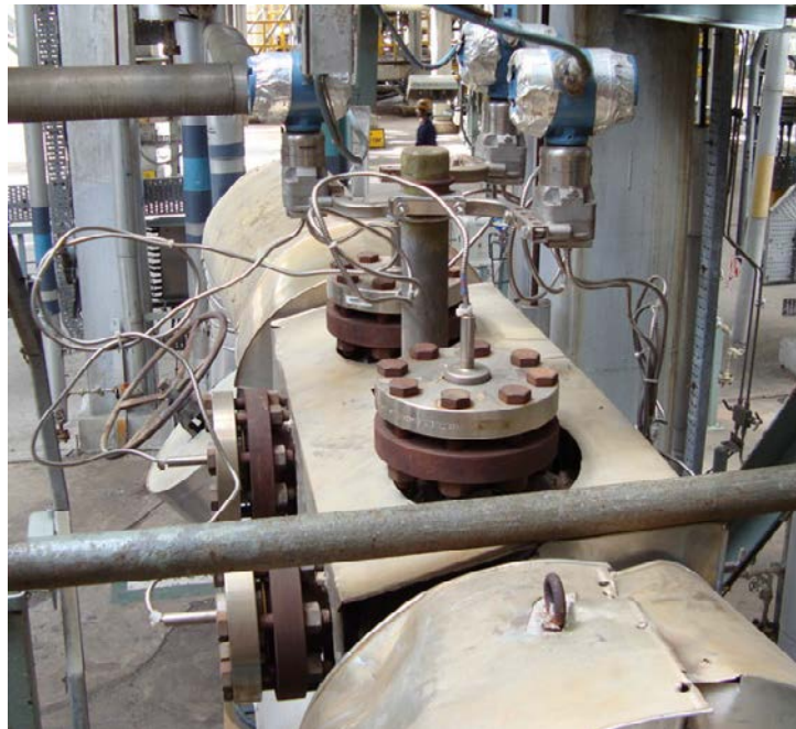
Fig. 3 : Wedge Flow Meter on Coker Feed Using Three DP Transmitters with Diaphragms
